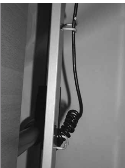
Wiring at the lifting motor, head end.
