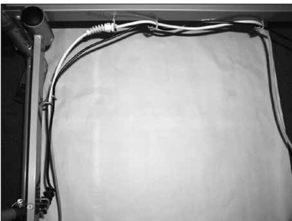
Wiring of the bed end motor (head).
