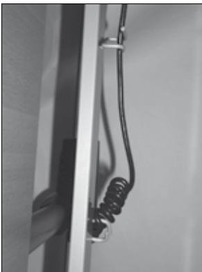
Wiring at the lifting motor, head end.
